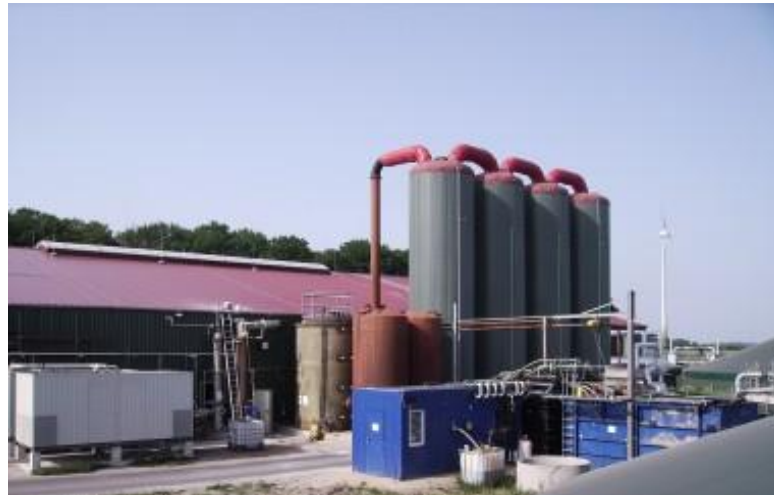
Large-scale strip system (BENAS) operating since 2008 , 15 m 3 /h flow capacity, testing of the FaserPlus-Technology, suitable for further technical experiments
